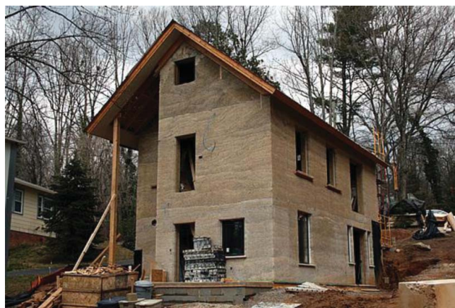
Figure 8. House insulated with hemp constructed in Asheville, North Carolina, USA. Photo courtesy of Clarke Snell.
