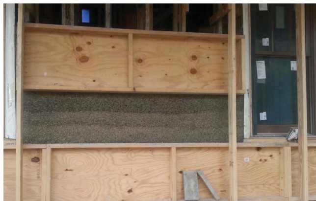
Figure 9. Cured hempcrete installed around framing timbers. Forms are set to pour the next layer of lime-hemp mixture. Photo courtesy of Carol Brighton.
